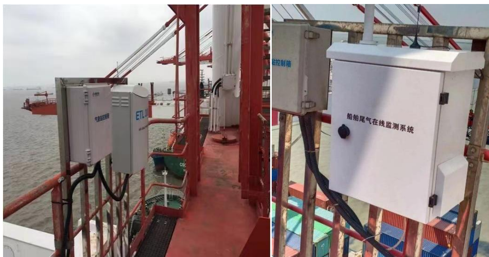
Figure 8- Quay drawbridge installation and deployment of shore-based fixed point reproduction monitoring equipment
