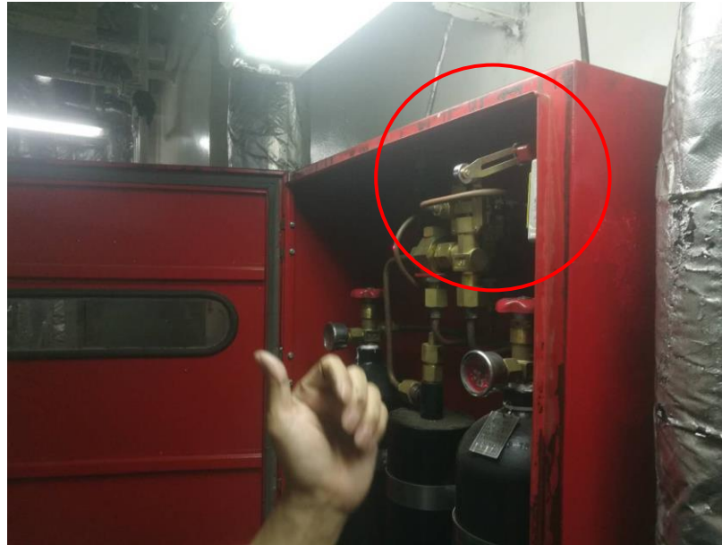
Figure 6 - Interlock device in CO 2 release control box Source: Author
