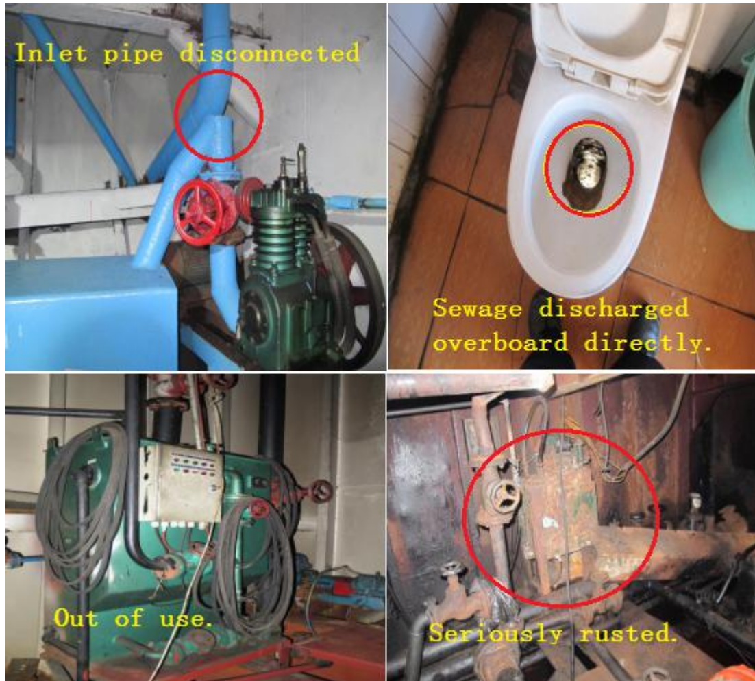
Figure 5.5 – Sewage treatment plant out of service. Source: Photos taken by the author during FSC inspection.
