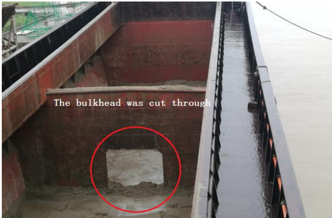
Figure 5.8 – Unauthorized reconstruction. Source: Photos taken by the author during FSC inspection.
