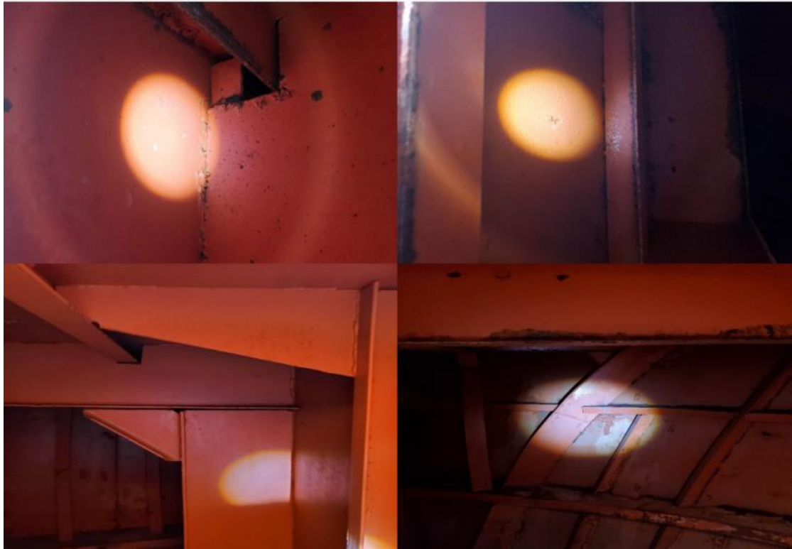
Figure 6.3 – Poor welding quality
